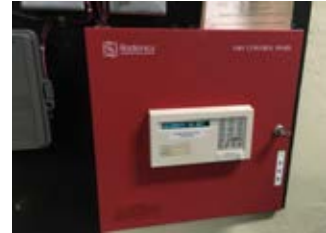
Boiler Monitoring System
