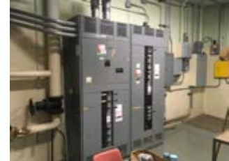
Main Electric Service
