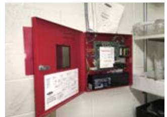
Fire Alarm System
